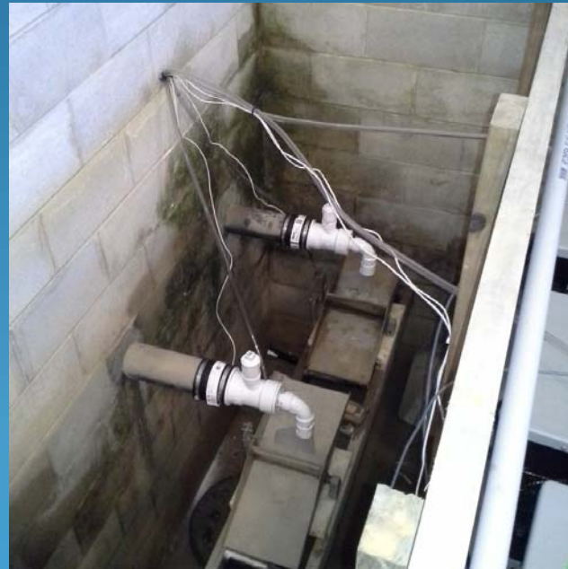
Tipping buckets, L-shaped pipes, connecting tubes
