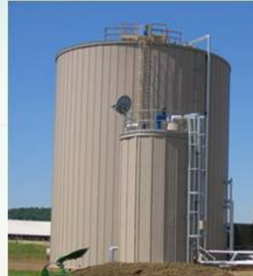
Complete mixed digester
