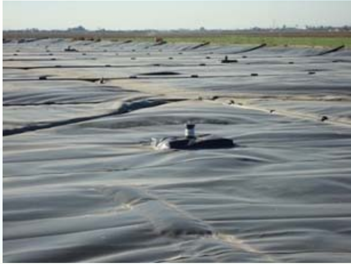
Covered lagoon digester
